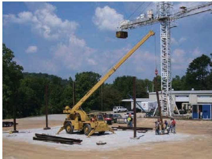
Boston Apprentice Kristi Canup operating the Grove Neckbreaker for the Steel Erection Class
